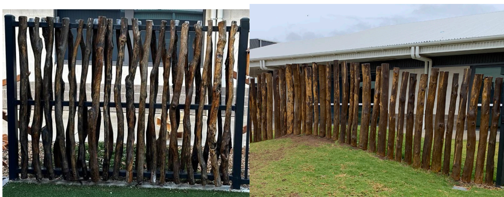
Figure 18: Examples of non-compliant fencing with entrapment risks.
